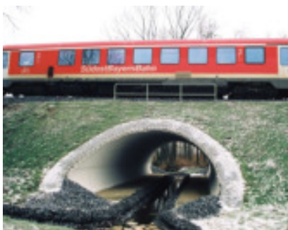
Picture 5: Culvert with double sidewalk for amphibians, small animals, etc.
